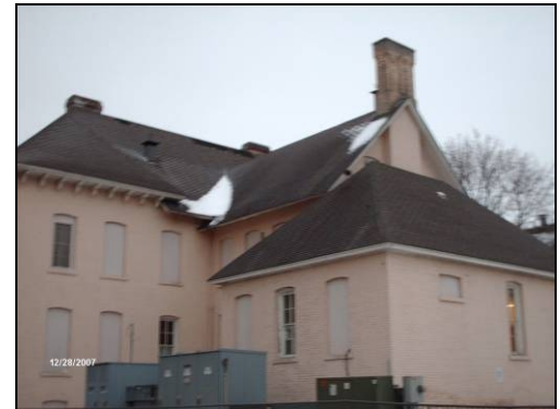
Deteriorated Chimney & Roof
