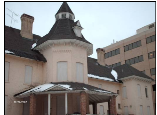
Deteriorated Canopy & Roof
